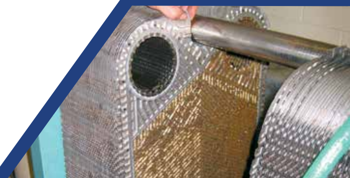
Protect Heat Exchangers
